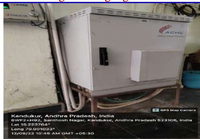
Server Rack-Principal's Chamber
