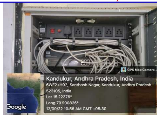
Server Rack-Computer Science Lab-2
